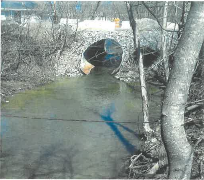
Figure 7. Undersized culvert on Sucker Brook on Lane Construction property.
