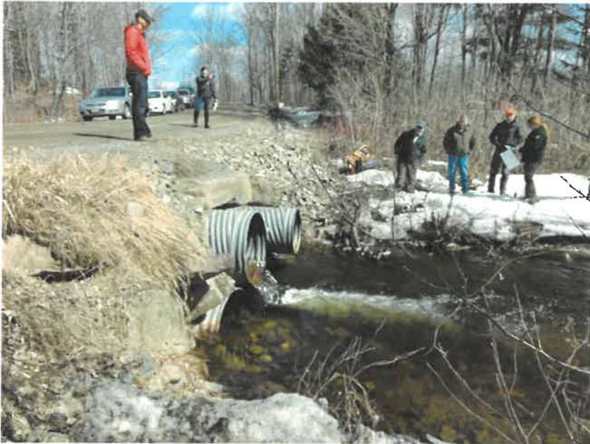
Figure 6. Perched and undersized culverts proposed for replacement at the crossing of Bacon Rd. over an unnamed tributary of Crooked Brook
