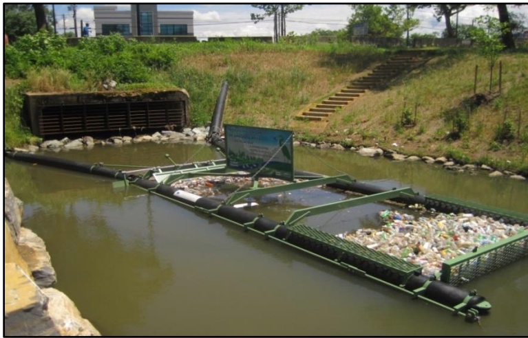
Figure 17. A Bandalong litter trap installed at the beginning of Nash Run, one of the District's tributaries to the upper Anacostia River (DC Department of Energy and Environment 2019).
