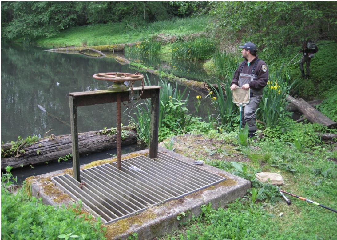
Figure 9. Water diversion structure and impounded area on Rinearson Creek within the Rinearson Natural Area restoration site. The structure is a passage barrier to upstream migrating fish. Five of seven 50 m GRTS sample reaches in Rinearson Creek were located upstream of the barrier.
